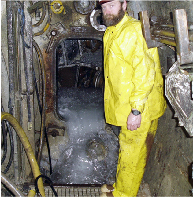
PHOTO: Water discharge through a shielded Tunnel Boring Machine's open pressure bulkhead, preventing maintenance and repair work. McMillen Jacobs Associates for the State of Michigan 11 .
